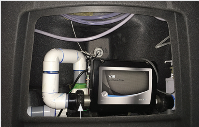
FIGURE 1.9a : HEATER UNION; LOOSEN UP TO BLEED AIR
